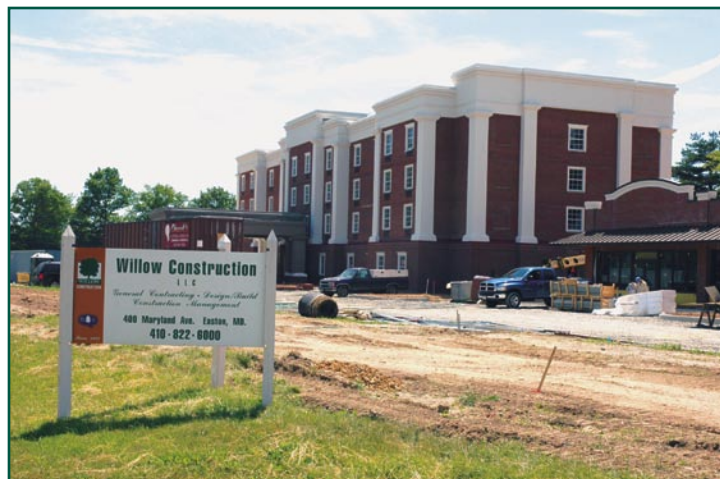
Willow Construction is the general contractor on the construction of the Hampton Inn on U.S. Route 50 in Easton.
